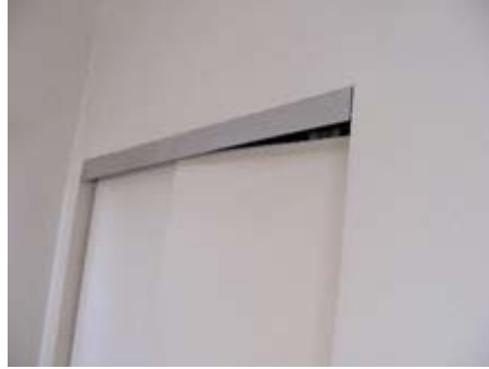
Closet Doors, Off Track
