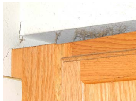
Improperly Installed Cabinets with Dust and Cobwebs
