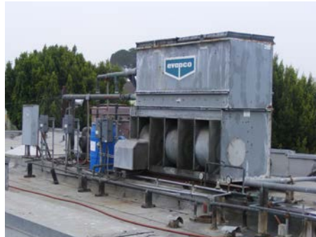
Cooling Tower and Hydronic Boiler
