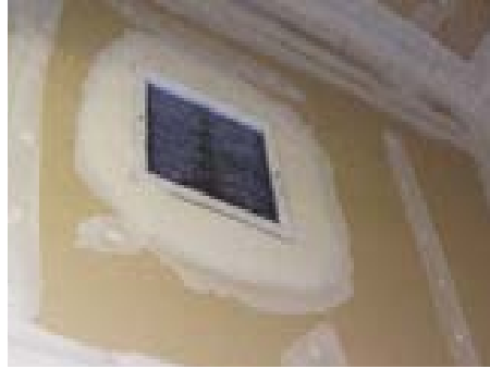
Sole Exhaust Grill In Elevator Room
