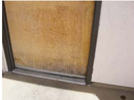
Damaged Entry Door
