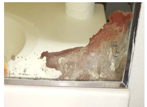
Damaged Vanity Mirror, Typical
