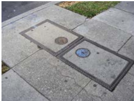
Water Mains in Public Sidewalk
