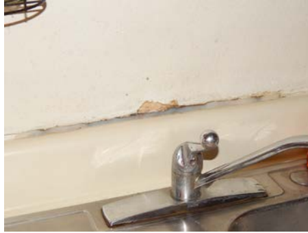
Water Damage Behind Sink
