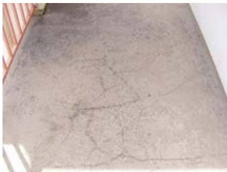
Cracked Deck Coating
