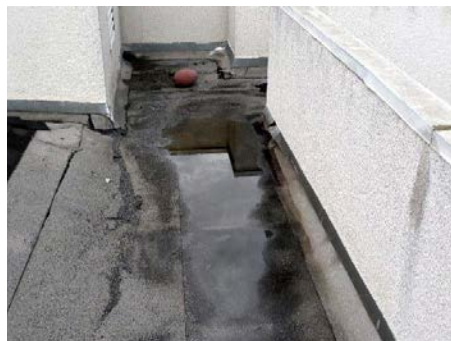
Weak Roof Sheathing w/ Ponding
