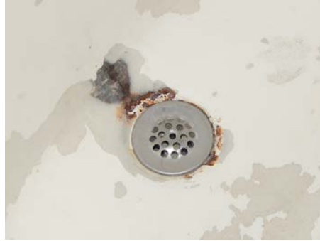
Damaged Tub Glaze w/ Rust
