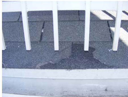
Damaged Roof Tile, Typical
