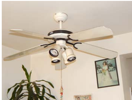
Ceiling Fan, Typical
