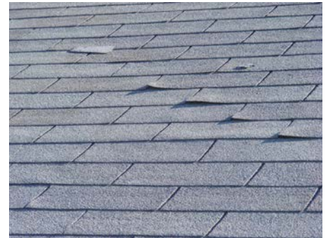
Peeling Roof Tile, Typical
