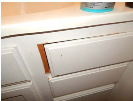
Damaged Vanity Drawers, Typical
