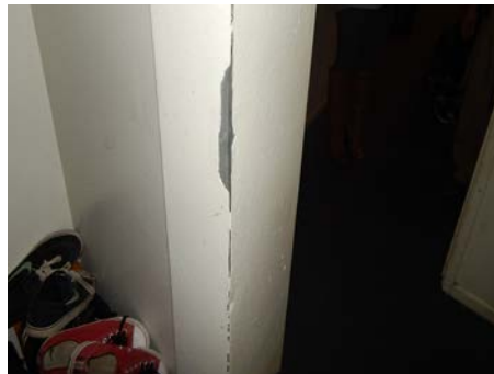
Damage at Corner, Typical
