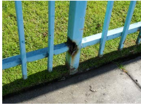
Rusted & Damaged Fencing
