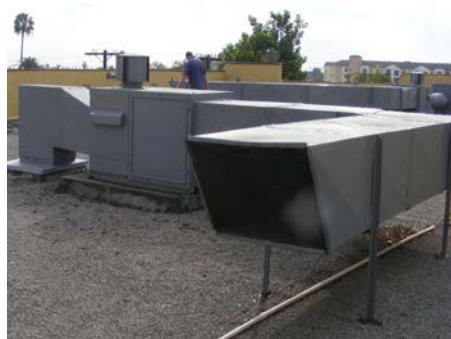
Roof Mounted Ventilation Equipment
