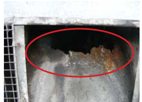
Rusted Fan Shroud on Cooling Tower
